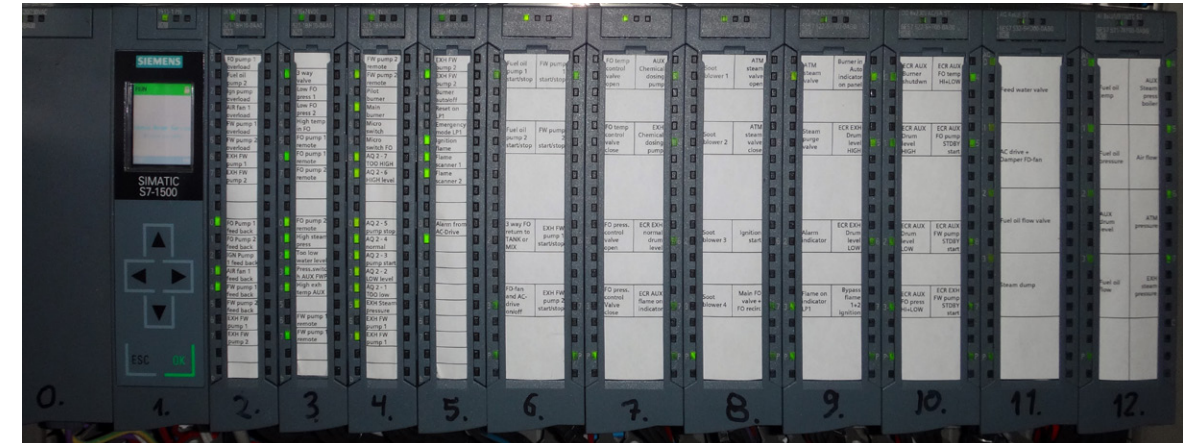
Figure 7: Complete PLC unit
