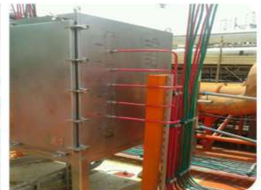
HYDRAULIC VALVE CONTROL SOLENOID BOX JACKET TUBING
