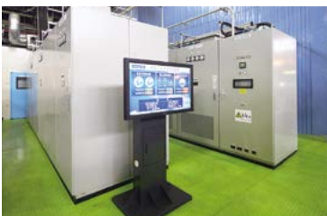
Power recovery system
