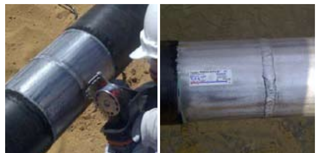
Surface preparation with Bristle Blaster®, result: thoroughly cleaned surface, also in pits, roughness 80 to 90 \mu\text{m R}_z (3.1-3.5 mils)
