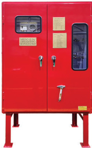
<Control box outside>
