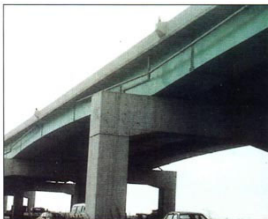
▲ DRAIN PIPELINES ON LARGE BRIDGE FOR VIBRATION-PROOF
