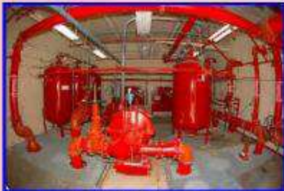
Foam System For Generator Room
