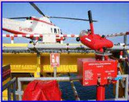
Helideck Foam System
