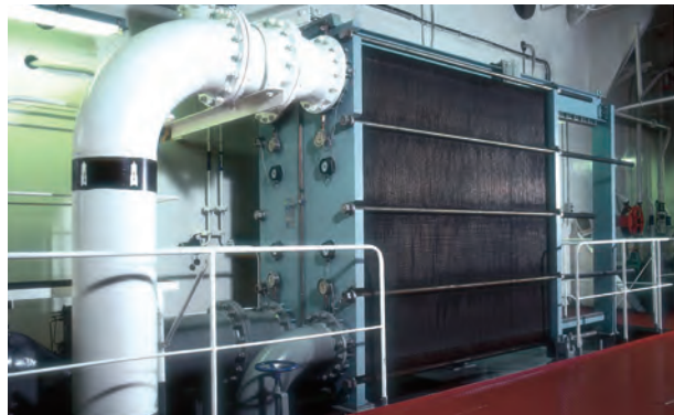
Main engine lube oil cooler
