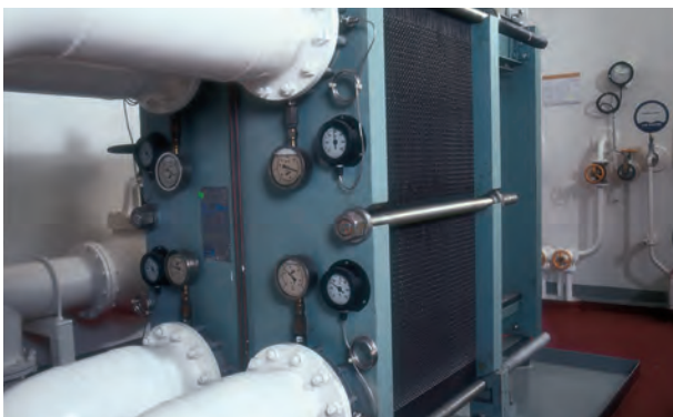
Jacket water cooler
