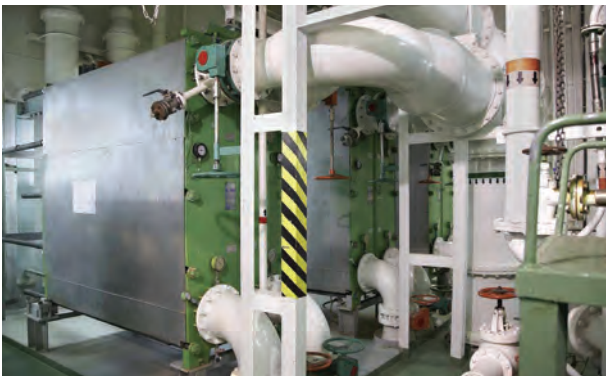
Central fresh water coolers
