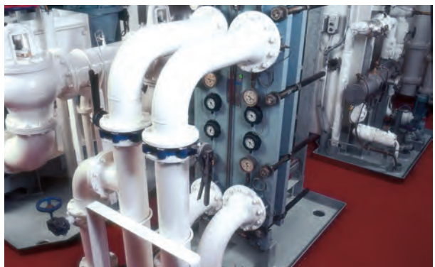
Stern tube lube oil cooler
