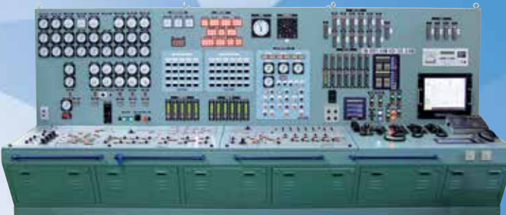
▲ Valve Remote Operation System Control Console
