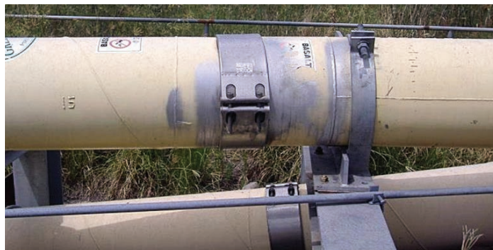
MJS EPDM 400A. mineral conveying line. Australia
