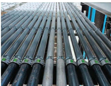
MGLP EPDM 50A, 80A, latex and coagulant conveying line, UPVC pipe, Malaysia
