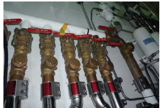
MJG NBR 40A. engine room. Taiwan
