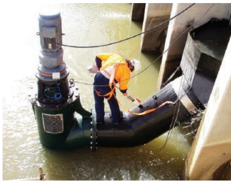
MJS EPDM 600A. hydroelectric plant. Australia
