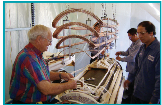
10 MW, 13.8 kV, 3600 RPM — generator rotor rewind
