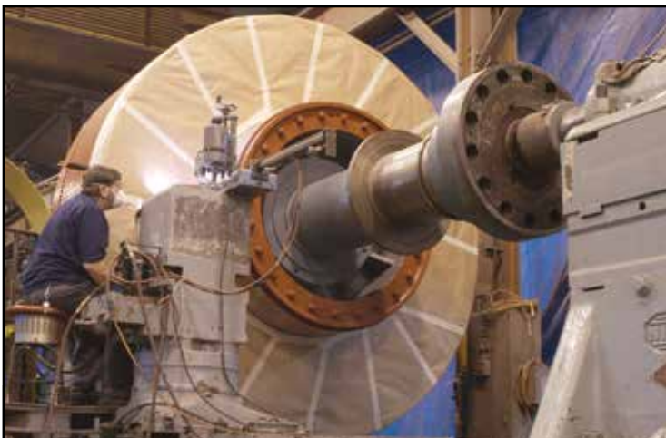
IPS technician profiles a large DC commutator.
