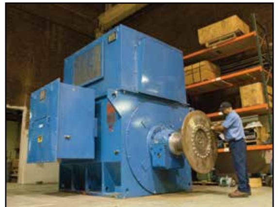
ID Fan Motor: 13,600 HP, 13.2 kV and 84,000 lbs.
