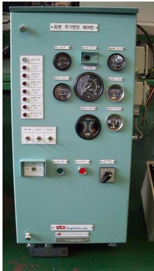
ENGINE CONTROL PANEL
