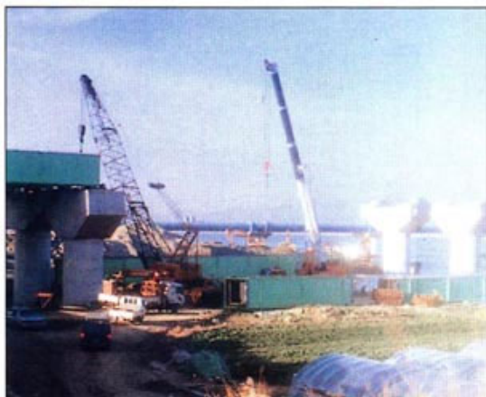
▲ LARGE WATER SUPPLYING PIPELINES
